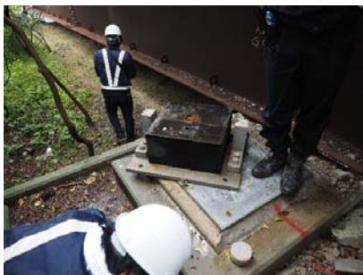
(c) 支承の損傷と桁のズレ
