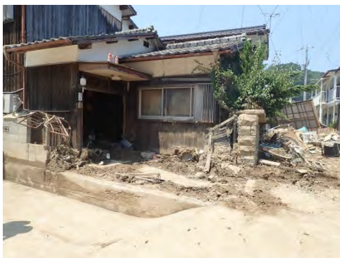
写真⑪(家屋崩壊)
