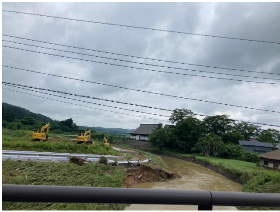
写真-2-12 護岸の洗堀と改修
