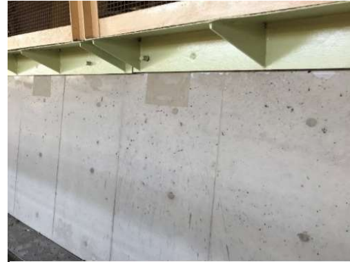
Example of the application of PolymerCrete to cross-sectional restoration of RC retaining wall inside a steel mill
