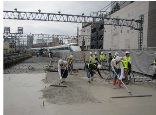
Concrete slabs for the railway track switching area at Tokyo Skytree Station
