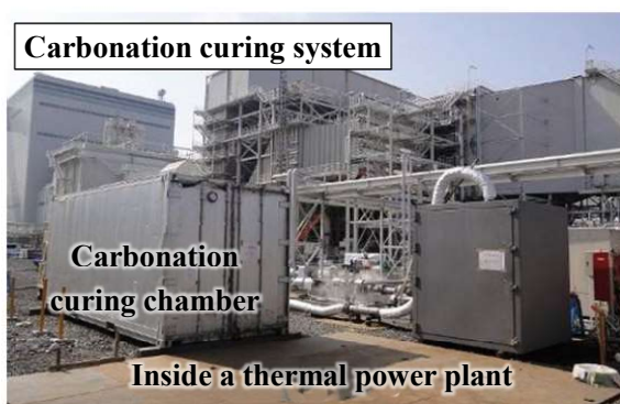
Figure 1.1 Curing tank installed at a thermal power plant
