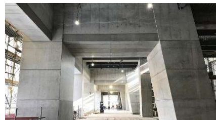
Use of Clean-Crete for the inside of the embedded formwork for erecting the girders that support the large roof of ES CON FIELD HOKKAIDO
