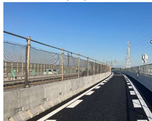
Temporary precast protection fence on the Yatomi viaduct of the Higashi-Meihan Expressway
