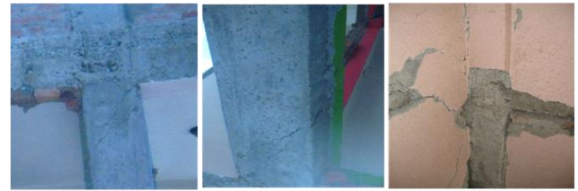
Column Damage Lv1
