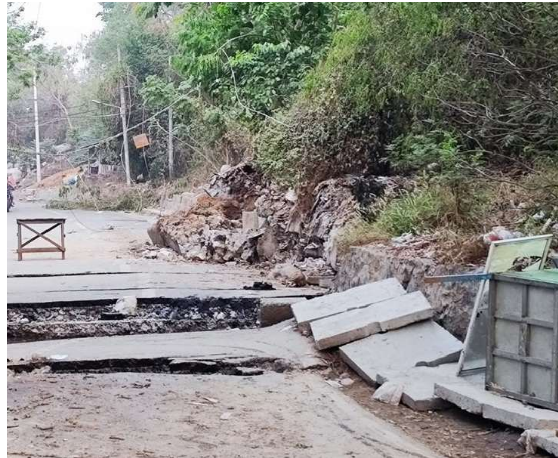
Slope and retaining-wall failures next to fault rupture
