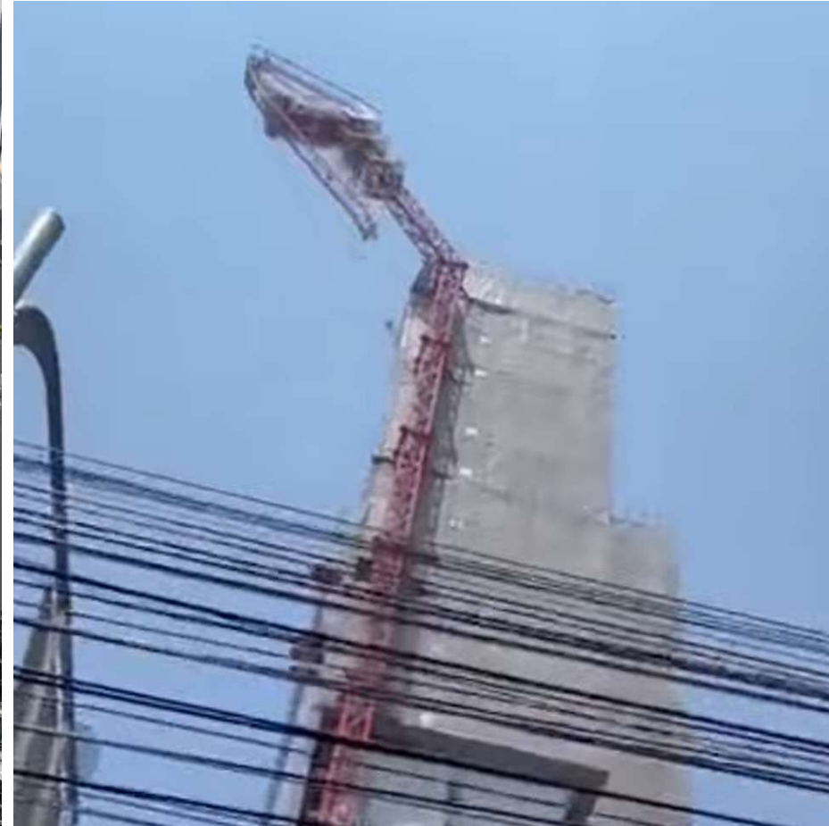
Collapsing construction Crain, Bangkok
