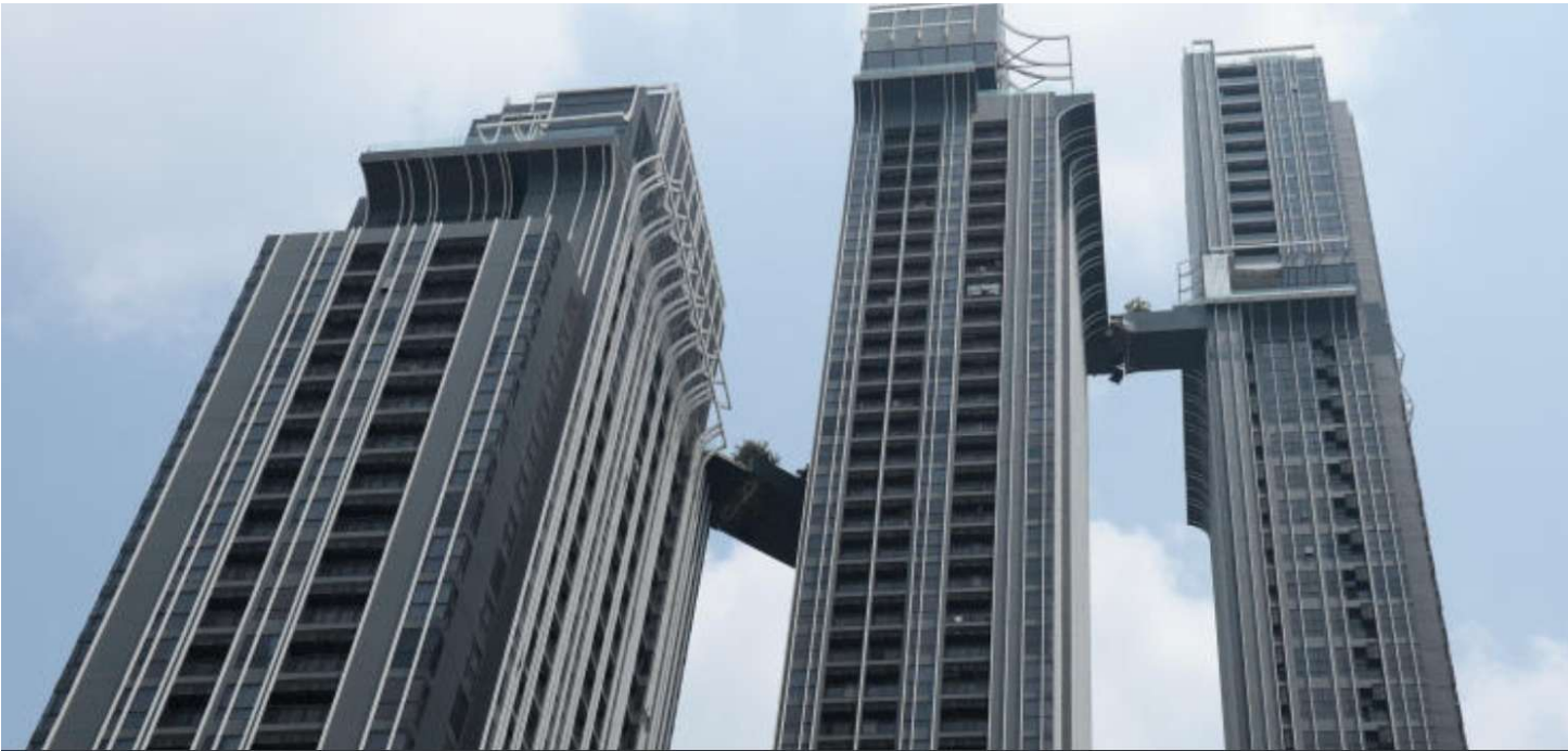
High-rise buildings with connection bridges damaged
