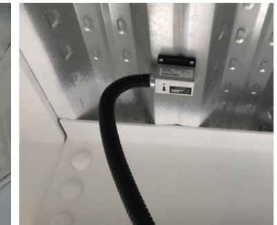
UA on ceiling
