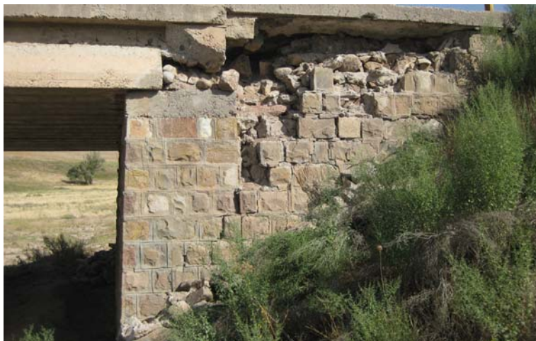
Damage to Abutment- West view
