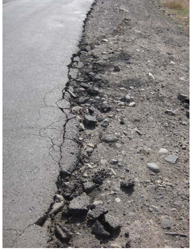
Cracks appeared due to landslides 100m after the bridge
