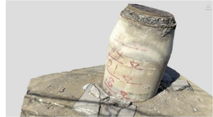
Lifted-up Manhole by Liquefaction
