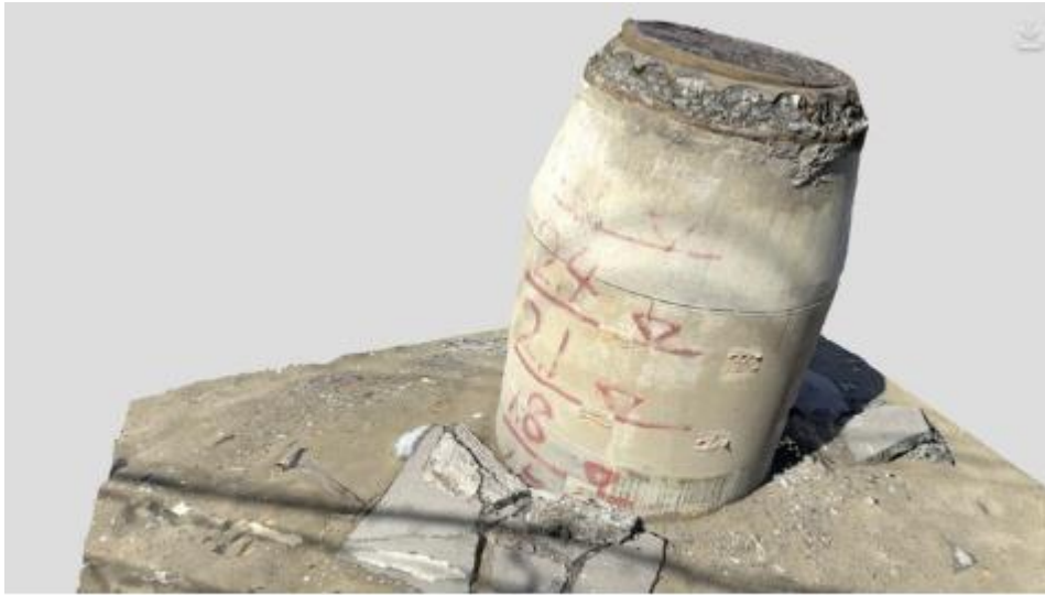
Lifted-up Manhole by Liquefaction
