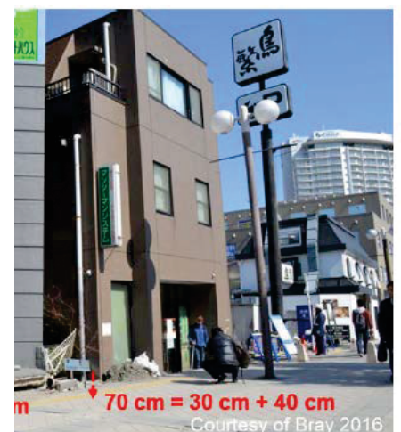
Building (Mat Foundation) -70cm Settlement
