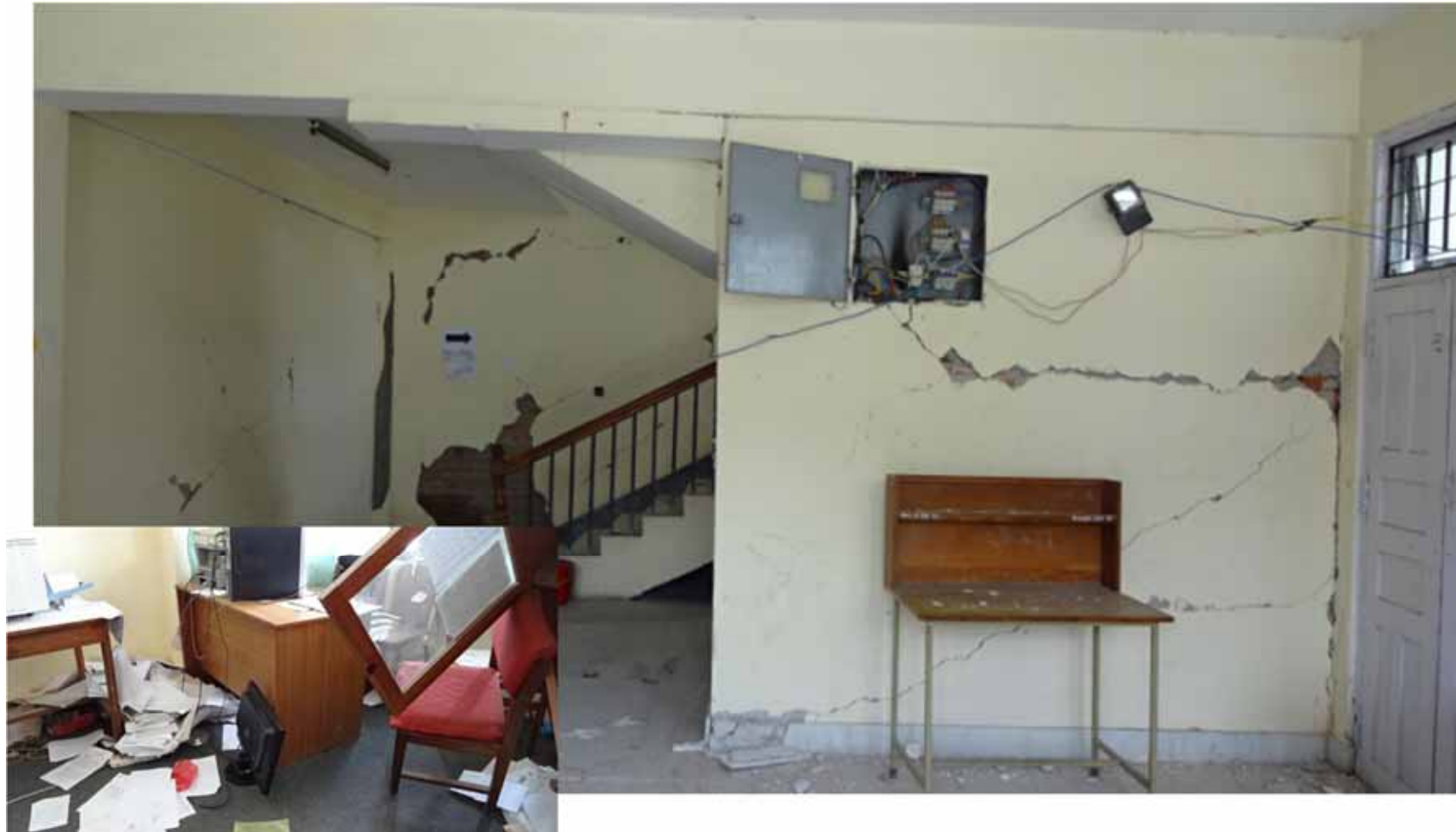
Brick shear walls suffered damage (G2). Subjects overturned (0.2g).
