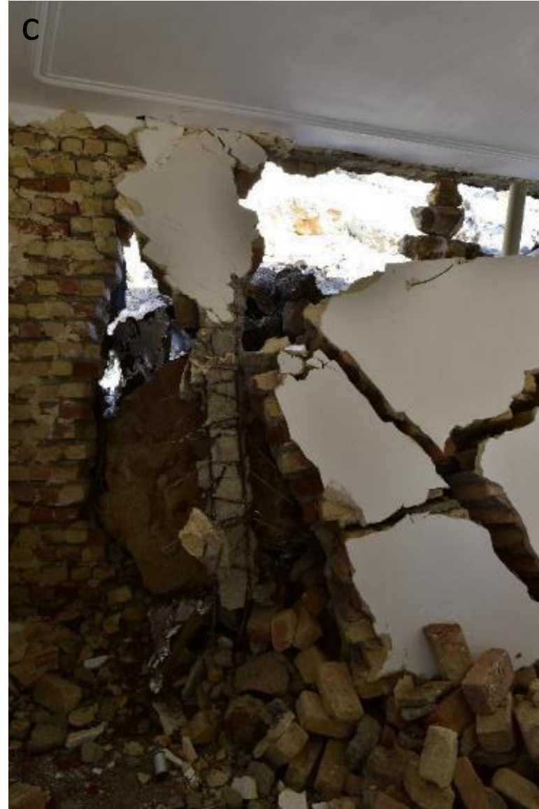
Fig. 18 (a,b & c) Damaged building due to landslides
