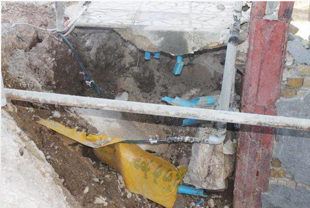
Damage to joints of the gas pipeline at the entrance to the houses at Ahmad-Abad town of Sarpole-Zahab city.
