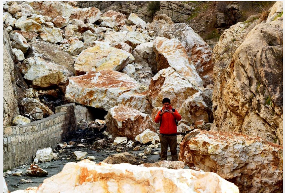
Severe rockfall at Ban-Zardeh Village road
