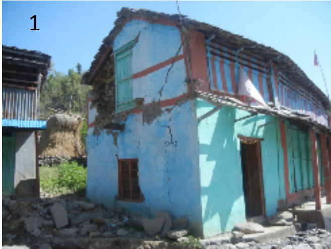
Typical damaged building
