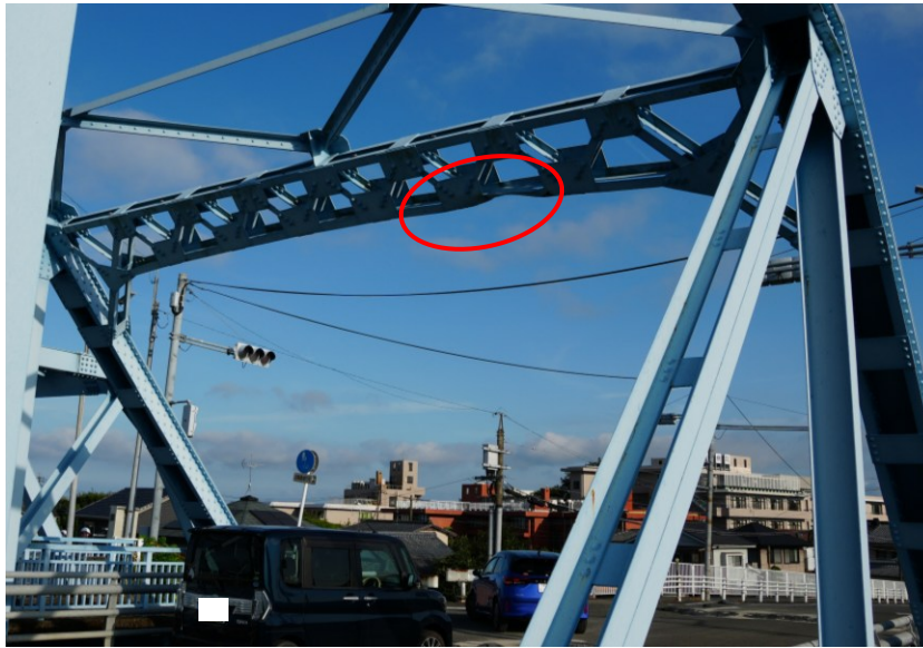
橋門構の座屈
