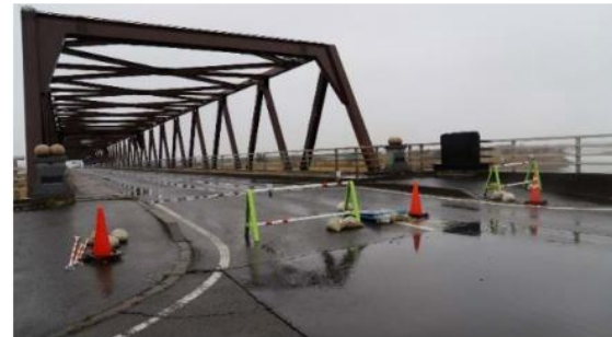
(a) The pavement cracked.
