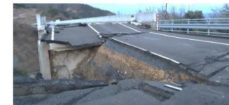
(c) Ground failure behind abutment
