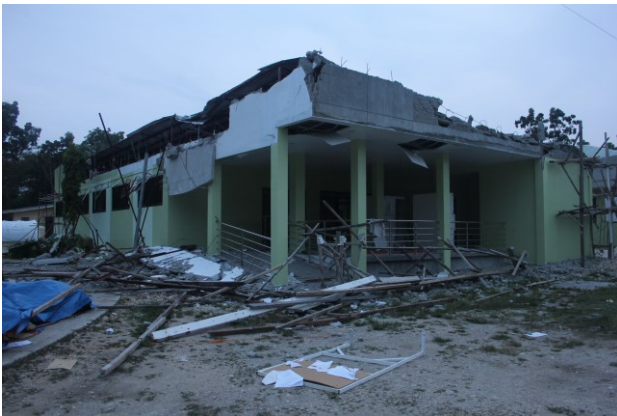
Fig.9 Structural damage to Natalio P. Castillo Sr. Memorial hospital.
