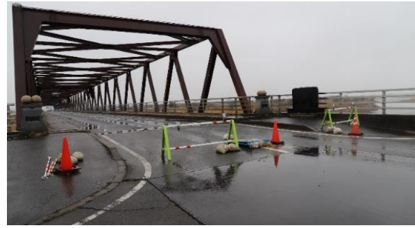
(a) The pavement cracked.
