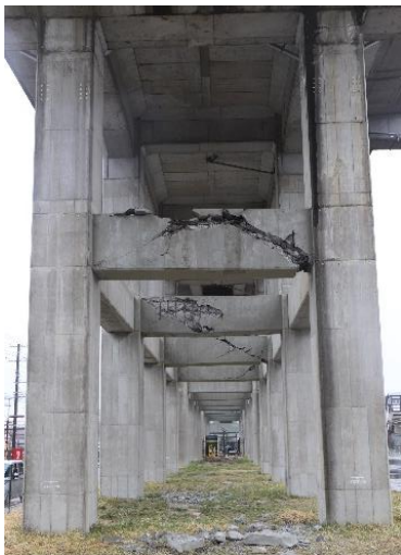
Photo.4 Shear damage to horizontal middle beams in Date City, Fukushima Prefecture. (37°49'30"N, 140°29'39"E)
