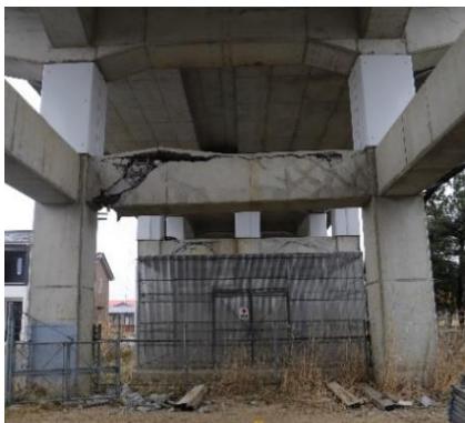
Photo.5 Shear damage to horizontal middle beams in Shiroishi City, Miyagi Prefecture.(37°59'33"N, 140°37'50"E)
