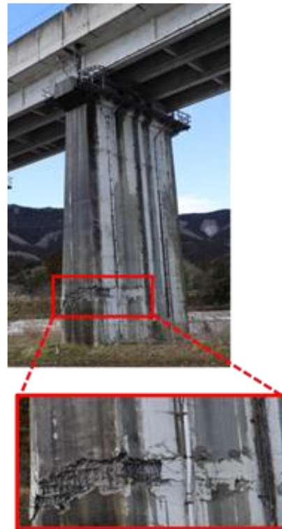
Photo.7 Flexure damage of RC pier in Shiroishi City, Miyagi Prefecture.(37°58'25"N, 140°36'54"E)
