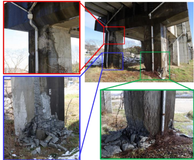
Photo.6 Flexure damage of RC pier in Shiroishi City, Miyagi Prefecture(Saikawa BV).(37°58'14"N, 140°36'44"E)
