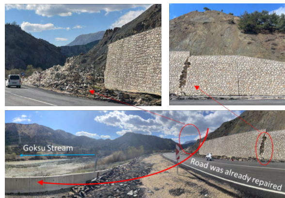
Fig. 23 On the Malatya-Golbasi Road: already repaired road embankment and damage of retaining wall (37.86332N, 37.76760E)
