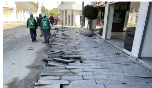
Fig.14 Sidewalk damage with the effect of liquefaction (36.58954N, 36.17355E).
