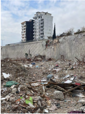
Fig. 7 A well-performed reinforced earth retaining wall with a damage occurred during the demolishing works of heavily damaged building nearby (37.57320N, 36.91964E).
