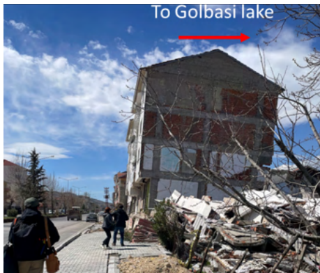
Fig. 2 Tilted houses in Golbasi, Adiyaman due to effect of liquefaction (37.79035N, 37.6519E).
