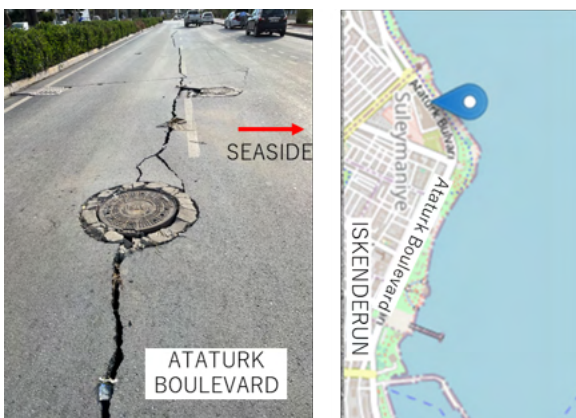
Fig. 12 Cracks along Ataturk Boulevard in Iskenderun due to lateral spreading.
