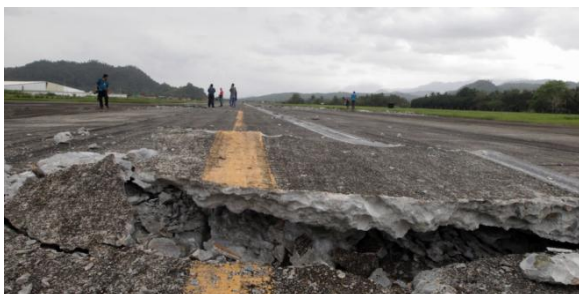
Fig.8 Damaged airport runway I Surigao del Norte.
