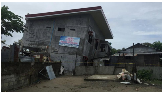
Fig. 4. Soft-storey column failure of a two-storey house.
