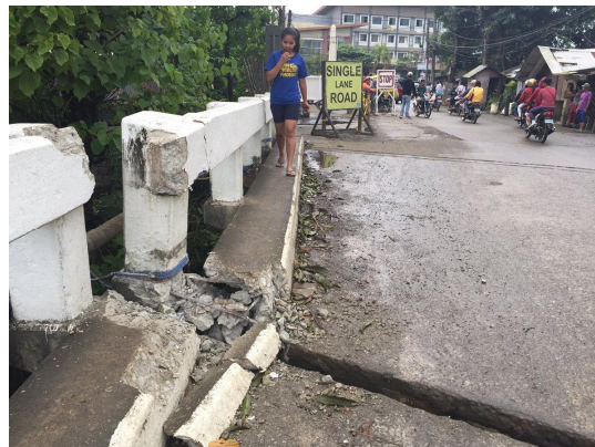
Fig. 6 Damaged to Malico Bridge.
