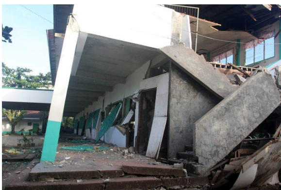
Fig 7. A damage building in San Nicolas in San Francisco, Surigao del Norte.
