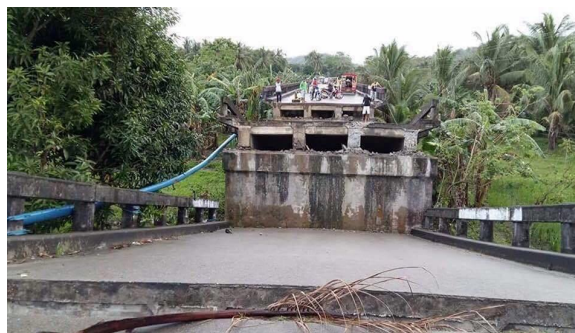
Fig.5 Failure of a Anao-aon bridge in San Francisco.
