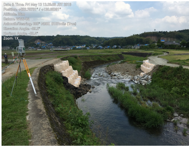
Fig.4 The terrestrial LiDAR setup and damage to the canal embankments. The main fault crossing is at the location of the repairs visible in the photograph.
