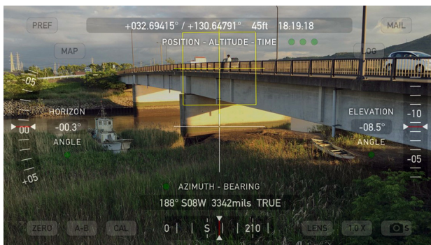
Fig.6 The Route 501 bridge that was not subjected to visible lateral spreading as would have been expected given the soil conditions at the site.
