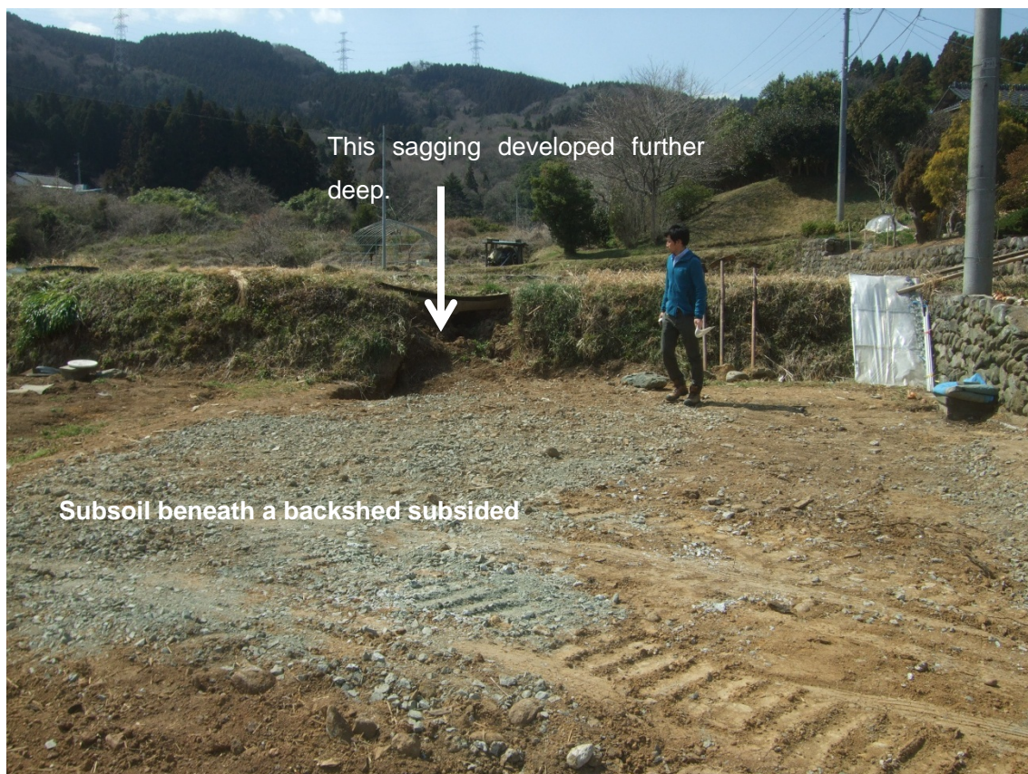
Fig. 4 Sinkhole (2m × 5m × 5m deep) at Tono plugged up (Photo by Kazuo Konagai at 36.994963, 140.729808 on March 27 th , 2012).
