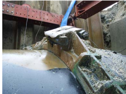
Photo 3 Sealing bolt worn out by hydro-blasting.
