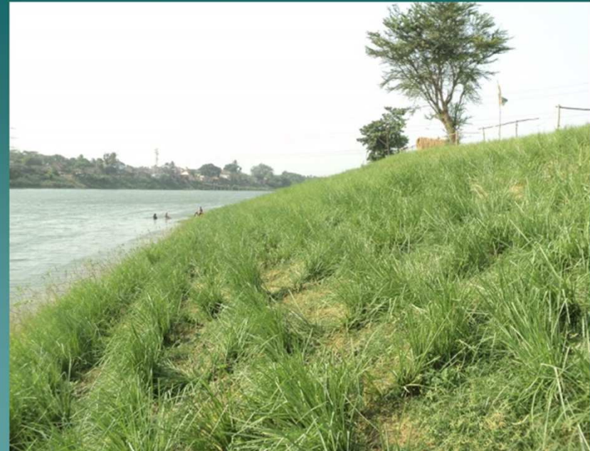
After plantation of vetiver at Udna, Tantishal G.P., for erosion protection of Mundeswari river, W.B.
