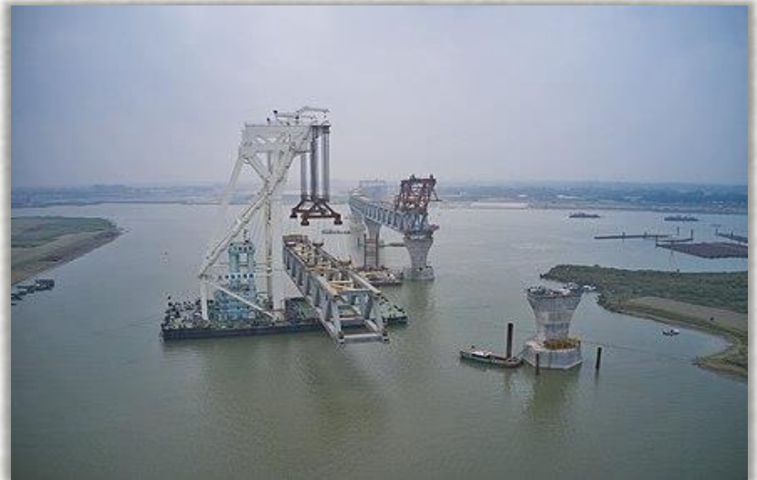
A view of the Padma bridge truss being lifted by Tian Yi Hao crane during construction
