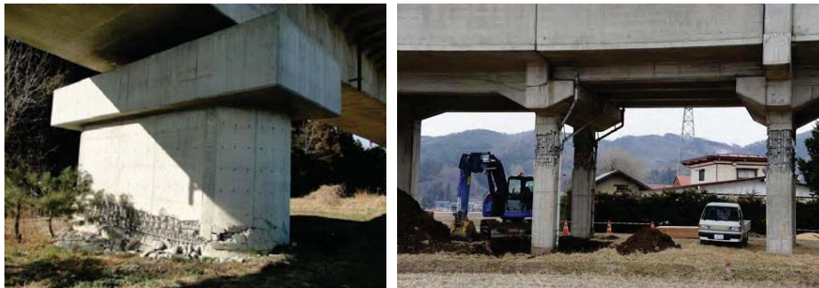
Damage of Highway Bridges Due to The 2011 off the Pacific Coast of Tohoku Earthquake (土木研究所資料)
