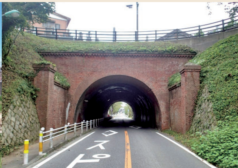
Seiso Railway No. 2 Tunnel, Chiba Selected as the JSCE Civil Engineering Heritage, 2014
