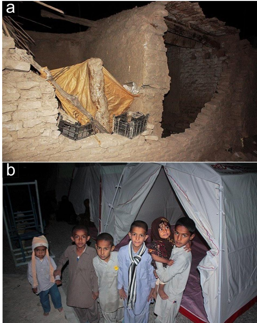
Fig. 2. a: Out of plane collapse of unreinforced masonry wall. b: Established tents of Iran Red Crescent near damaged people [6].
