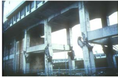
1995 Hyogo-ken Nanbu Earthquake
