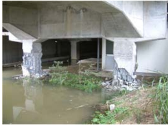
2004 Niigata-ken Chuetsu Earthquake
